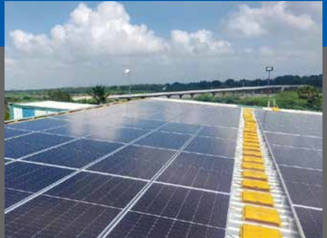
680 kWp Daniyawan, Bihar
