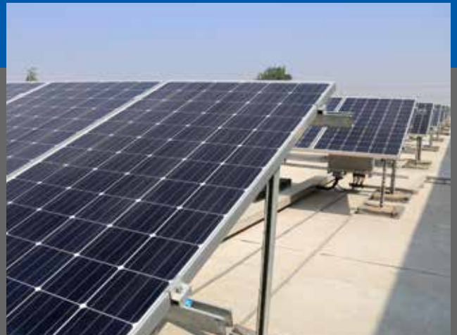
800 kWp Sriperumbudur, Tamil Nadu
