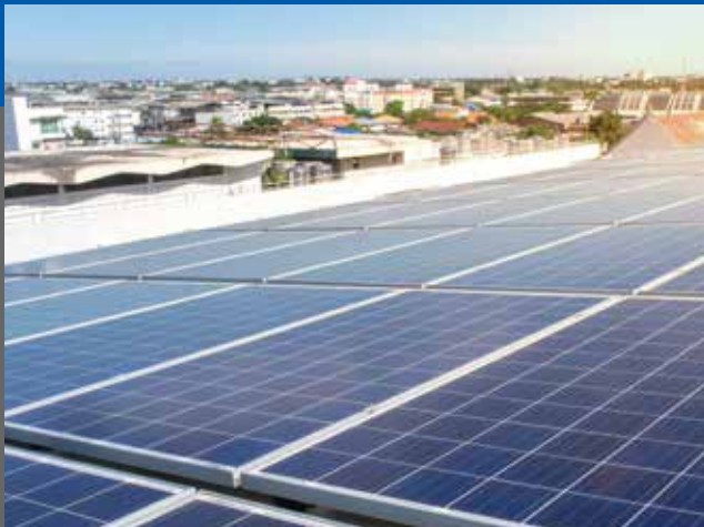
1 MWp Hyderabad, Telangana
